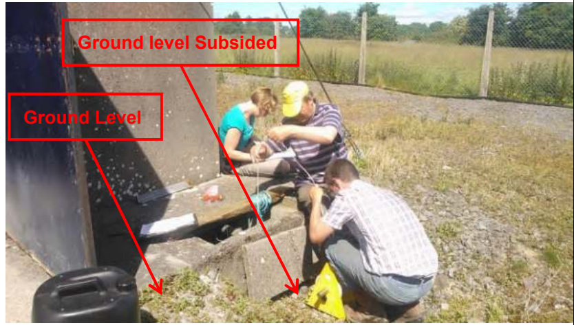
Photo 4: Borehole Chamber – Note the Dip in ground level adjacent to chamber due to subsidence
