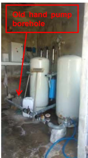
Photo 3: Rusheens GWS - Pumphouse (Internal)
