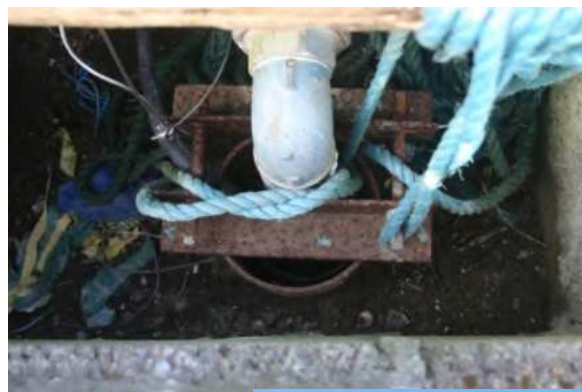
Photo 6: Well head inside borehole chamber showing 150 mm steel casing and rising main
