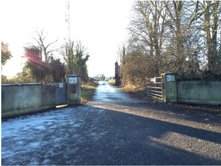
Plate 29: Entrance to existing Cloon 110kV substation.
